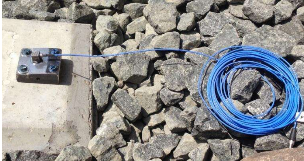
Figure 2.2. A PCB 356A01 triaxial accelerometer installed at the Portal
