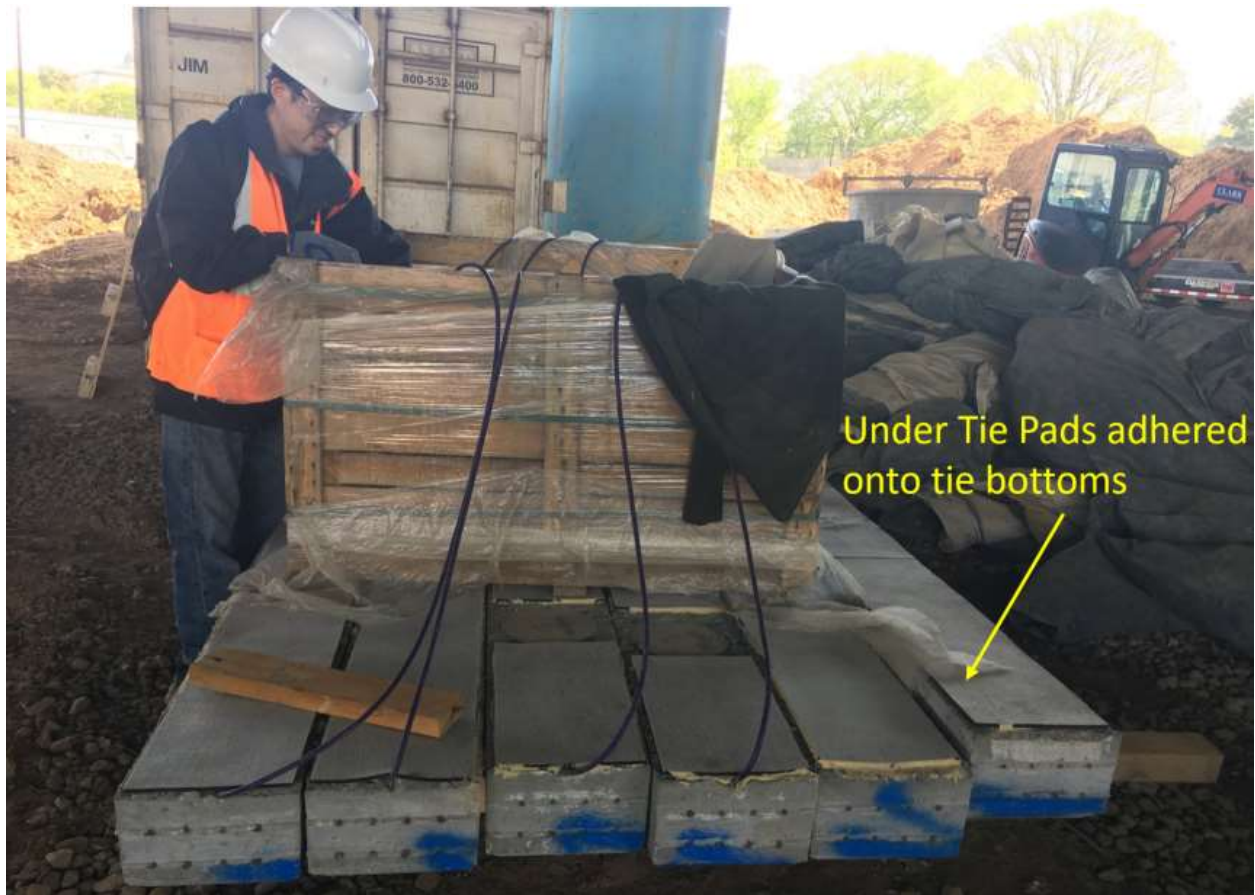
Figure 1.8. Instrumented prestressed concrete ties with the tie bottom side up showing the UTP at the tunnel storage yard before installation, with sensor wires protruding from the ties and stored in a crate on top of the ties
