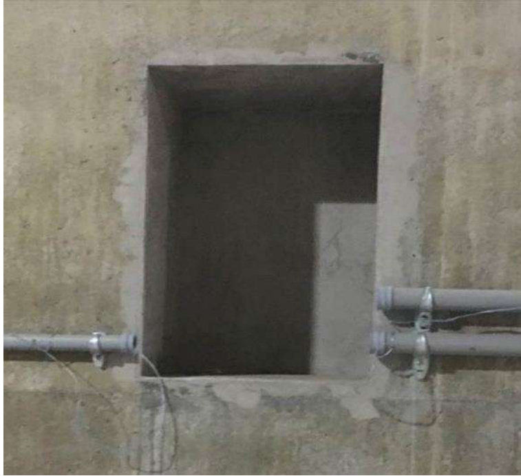
Figure 3.2. View of a recess used for the data acquisition cabinet at Station 23
