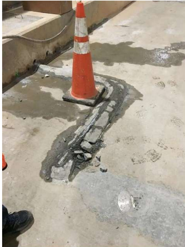
Figure 4.2. Pressure sensor grouted into block out in the tunnel floor with sensor cables protected and run to the walkway hand hole
