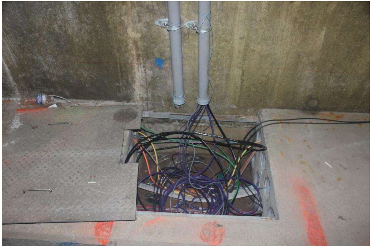
Figure 3.3. View of cables passing through recess under the walkway to the conduit leading to the data acquisition cabinet
