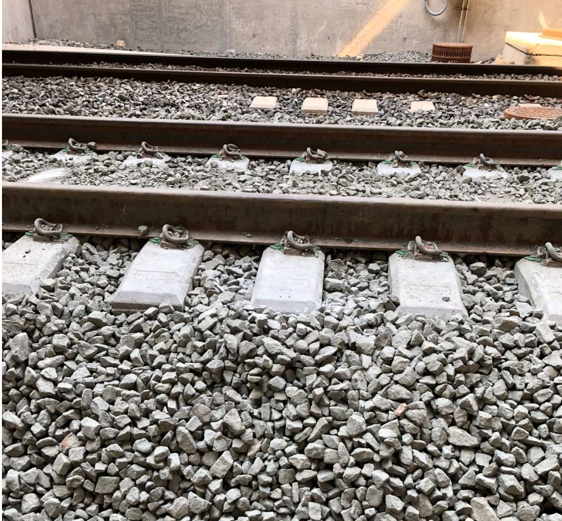
Figure 1.2. Rail at the west entrance to the tunnel showing the rail, prestressed concrete ties, fastener system, and ballast
