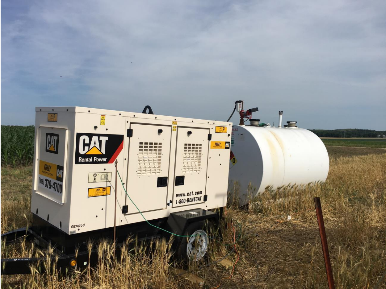
Appendix A Figure - 2 Caterpillar XQ35 Generator and 3,785-liter diesel tank
