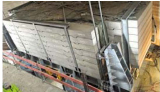
Fig 2 The installed ATMD
