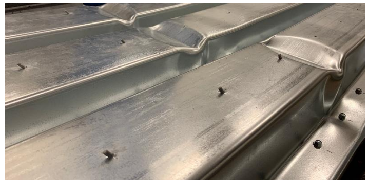
Figure 14: Post-test showing plastic mechanisms in top deck and sheared screws between panel and top flute of top deck
