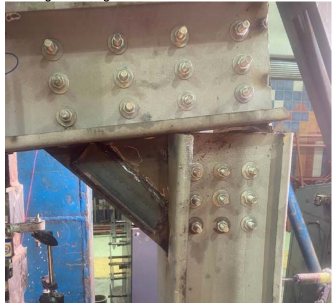
Figure 11: Tearing in the gusset plate observed in S2
