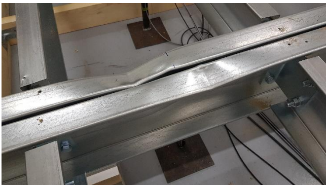
Figure 16: Failure mode of middle double primary beam
