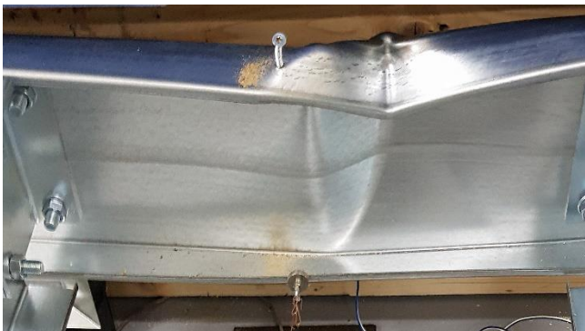
Figure 18: Failure mode of outer single primary beam
