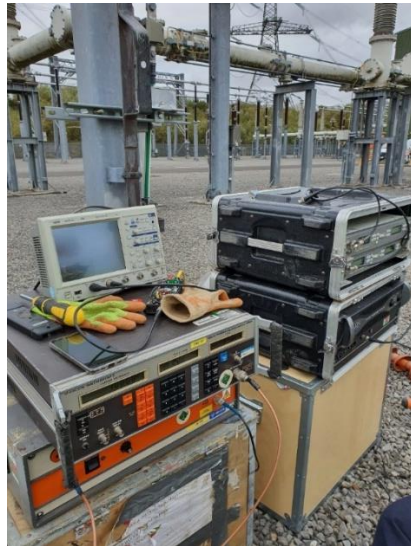
Figure 7.24: Earthing measurement setup at Substation ‘A’.
