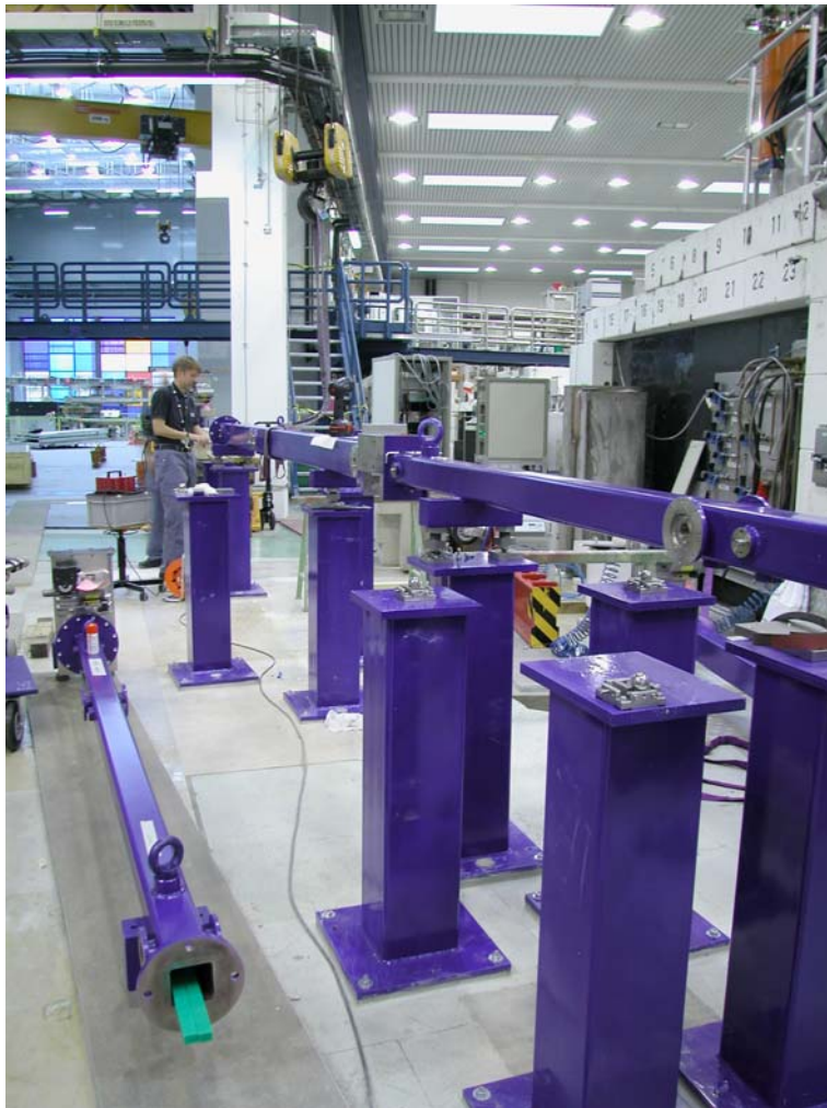
The neutron guides leading from the reactor to the instruments in Neutron Guide Hall 2 are being installed.
