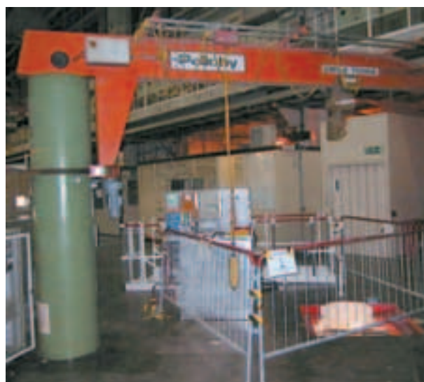
Figure 2. Top floor of the INES instrument showing the crane, the service panel and the opening in the floor that will accept the sample cage.
