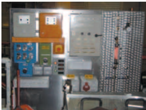
Figure 3. View of the service panel with the interlock system keys (A), the CAMAC serial plugs (B) and the helium lines for cryogenic applications (C).
