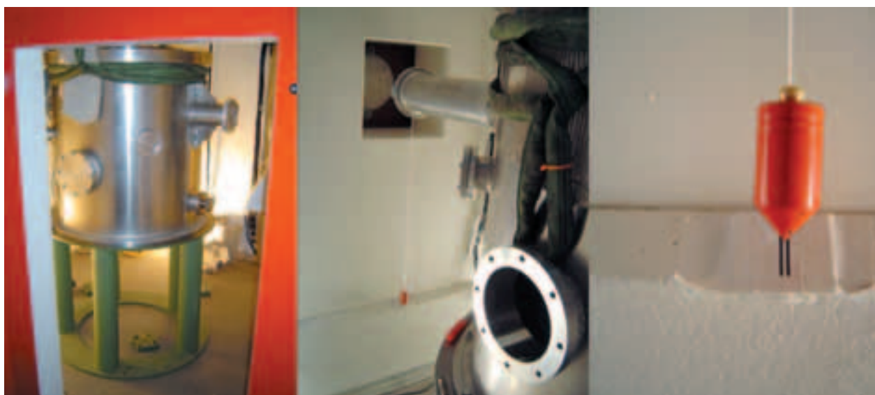
Figure 5. Sample container and frame (left). Positioning and proper orientation of the sample chamber using a plumb line and the reference points marked on the walls (centre and right).
