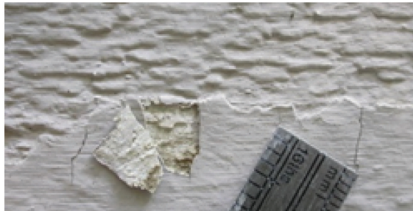
Figure 4: Fungal growth into painted surfaces (source: www.InspectApedia.com ).
