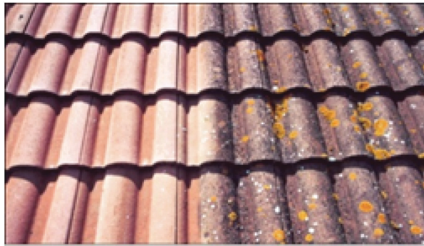
Figure 1: Roof shingle soiled by lichens and pollutants (courtesy of John Gillat, Thor Specialities –UK Limited).
