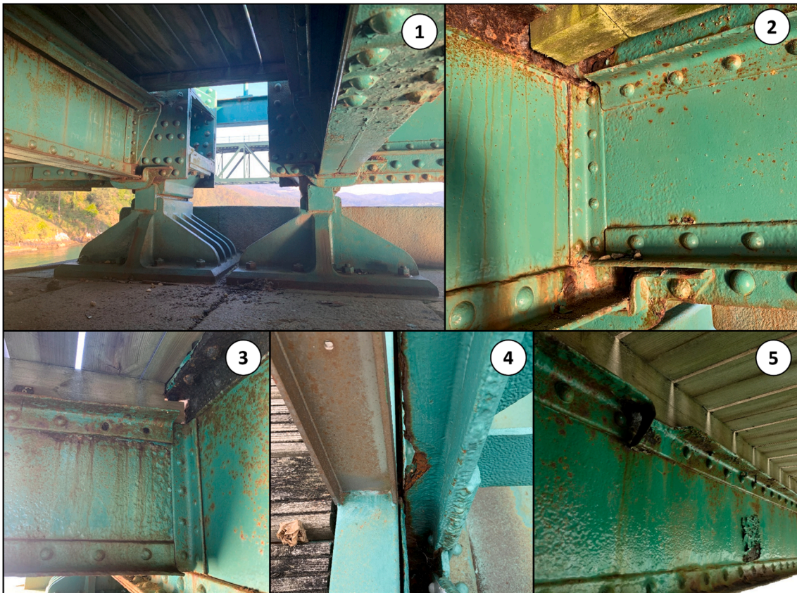
Fig. 7. Details of the current condition state of the bridge: (1) simple support and the gap between spans (2) connection between stringers and crossbeams (3) lack of rivets in a stringer (4) heavily corroded retrofitted vertical hanger (5) corrosion in a crossbeam.
