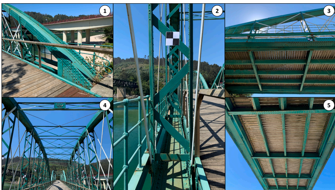
Fig. 5. Details of O Barqueiro Bridge: (1) arch rib (2) vertical hanger (3) stringers (4) sway systems (5) crossbeams.
