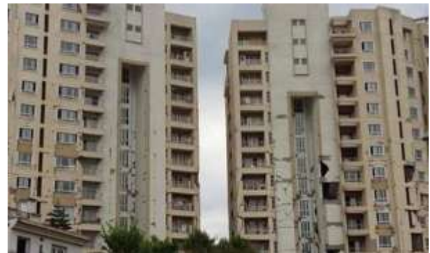
Fig. 5 Shear failure in masonry wall after earthquake in Nepal [11]
