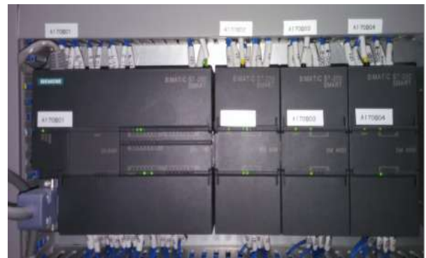
Fig 6: A complete view of the PLC along with the Analog and Temperature modules.
