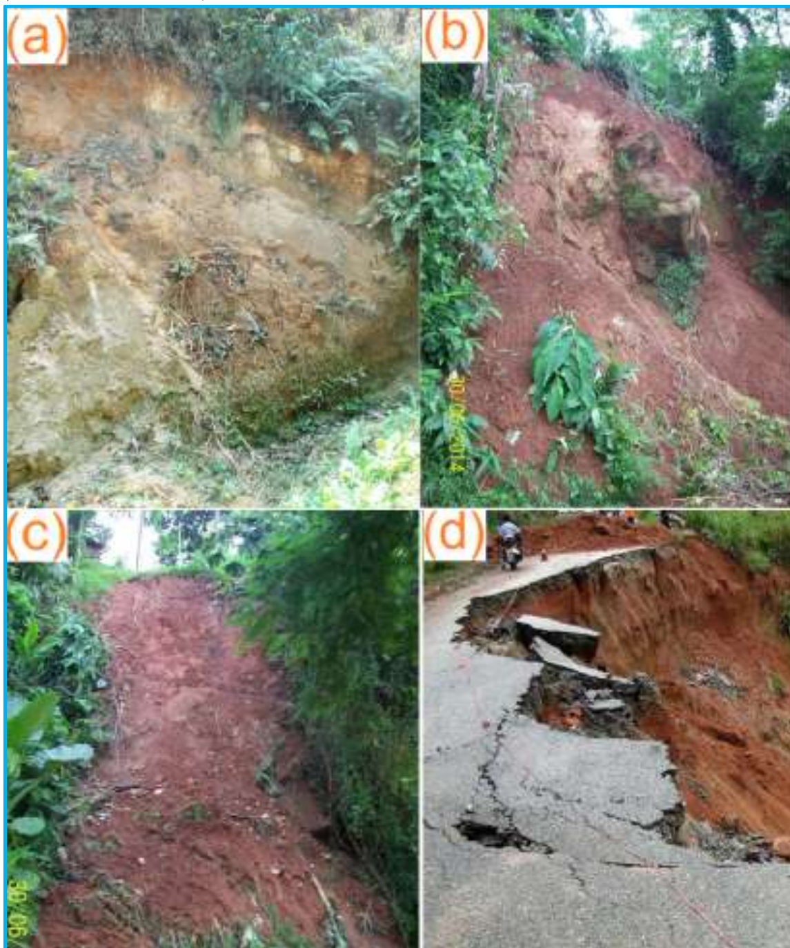
Figure 3: Photos of landslides within the study area: (a) Incipient Translational Slide; (b) Translational Soil Slide; (c) Translational Soil Slide; (d) Roto-translational Slide, which caused the destruction of a road
