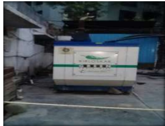
Figure.No.4.5 Diesel Generator
