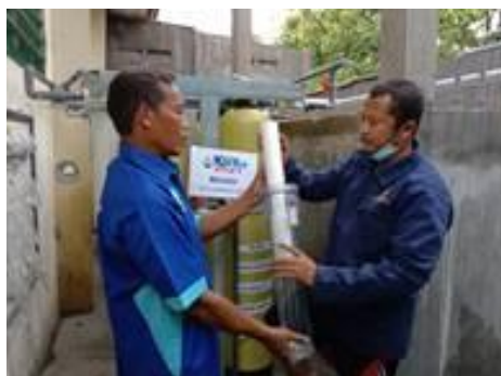
Gambar 6. Pencucian Housing Filter
