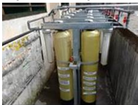
Gambar 5. Pencucian Housing Filter
