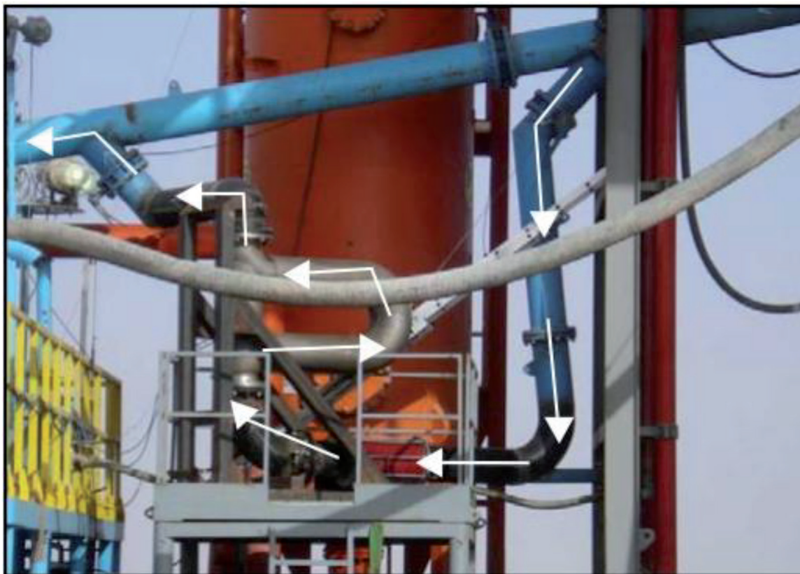
Figure 2. Coriolis installation on the bell nipple of a conventional drilling rig. N.B.: The arrows indicate the bypass and flow direction through the Coriolis from bottom to top [26].
