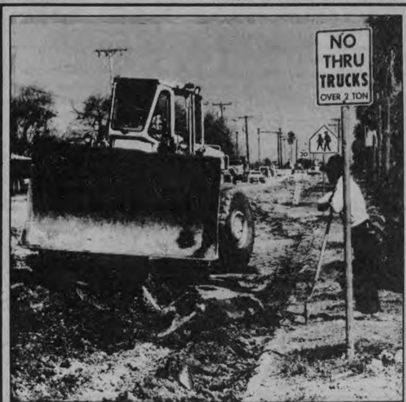
Rain during the Christmas holidays has delayed completion of the Sugar Road drainage improvement project by at least a month.
