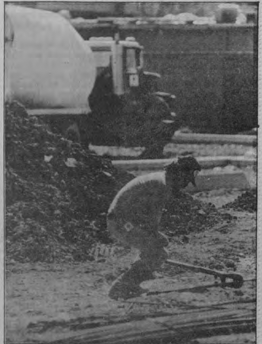
Construction continues—A worker cuts reinforcements for the driveway around the new Communications Arts and Sciences Building. Problems with the soil around the building caused delays because a spanning cloth had to be laid. For more information see story elsewhere on this page. (Photo by Delcia Lopez)
