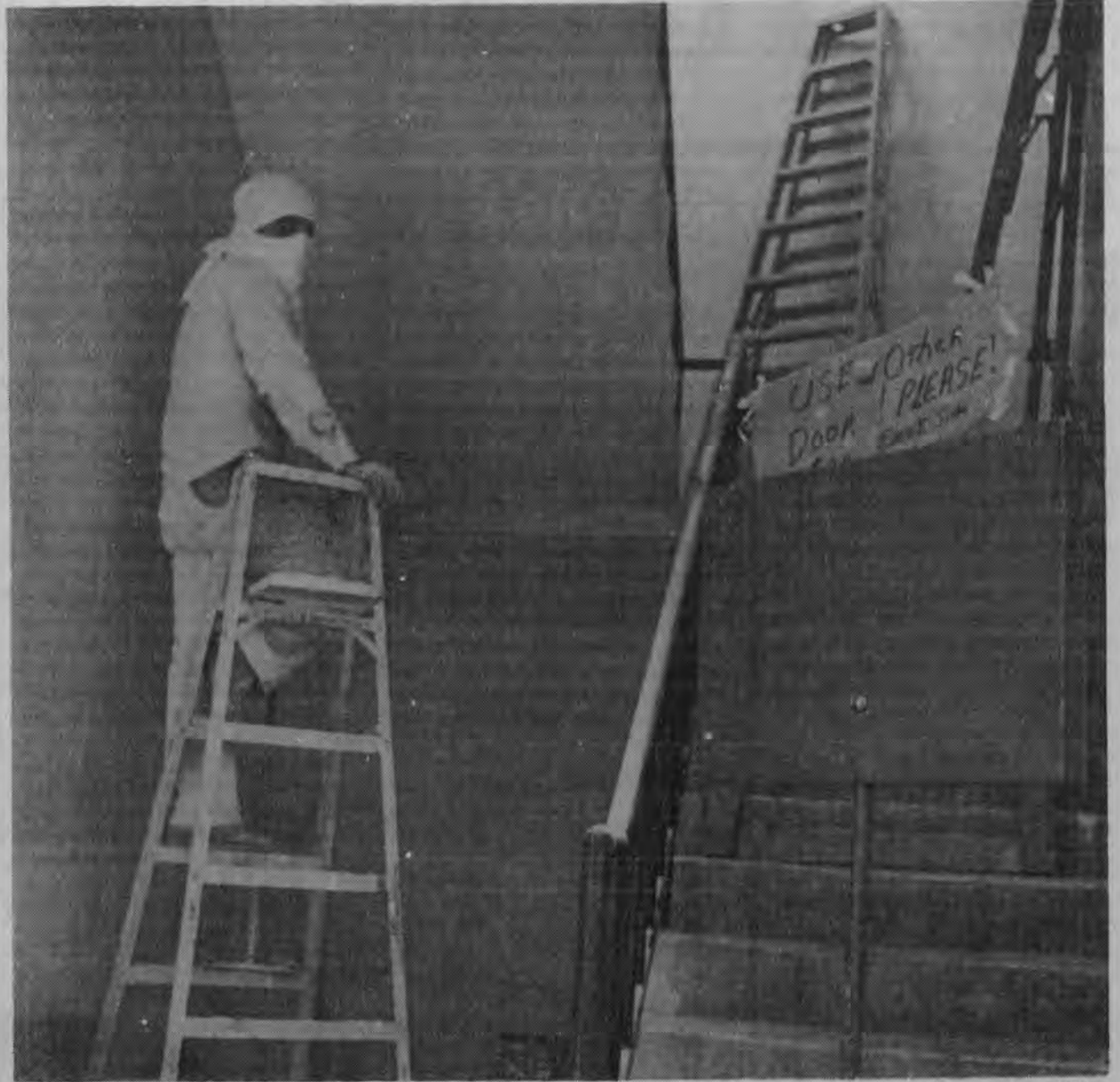
Do I need a gas mask, too?--Hazardous materials necessitate the use of air filters by this construction worker of the yet unfinished Communications, Arts and Sciences Building. (Photo by Delcia Lopez)
