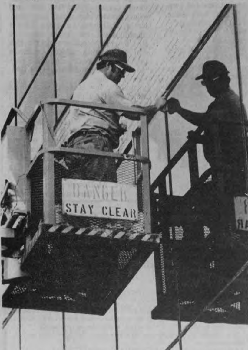
A Helping Hand--Ronald Champagne had a little help from his shadow while sealing the expansion joints on the windows of the Liberal Arts Building. (Photo by Jesse De Leon)
