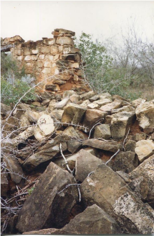
Sandstone structure in ruins.
