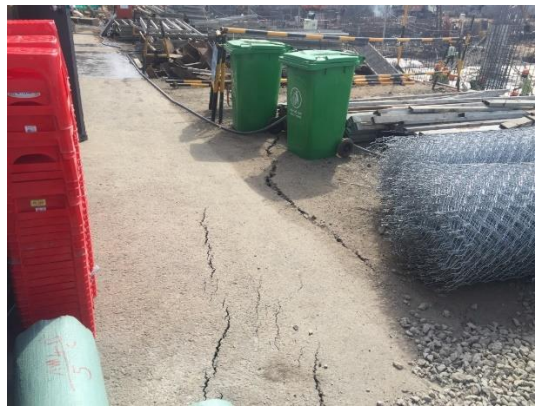
Figure 6. Road with soil cracks near the excavation
