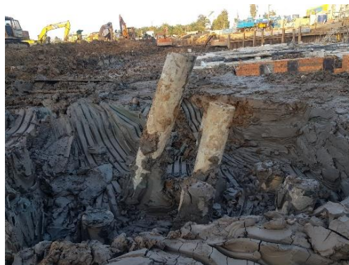
Figure 4. Pile displacement at Axis B during excavation
