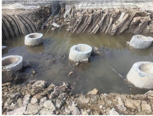
Figure 5. Pile displacement at Axis A during excavation
