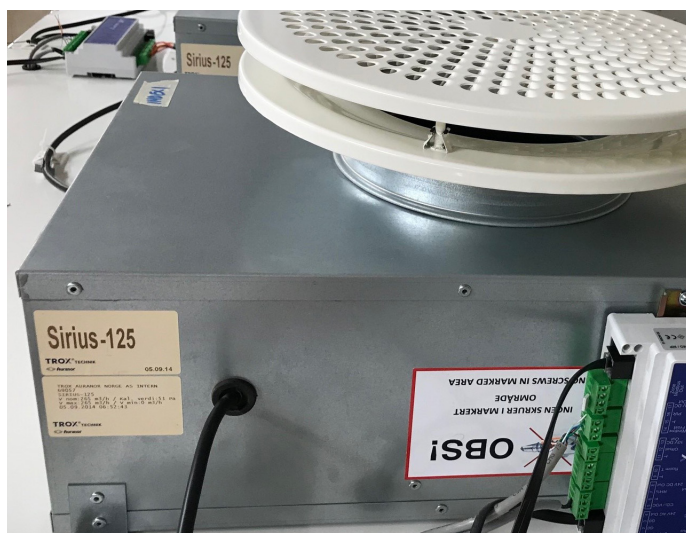
Labelling of plenum box and terminal device. Photo: SINTEF Community
