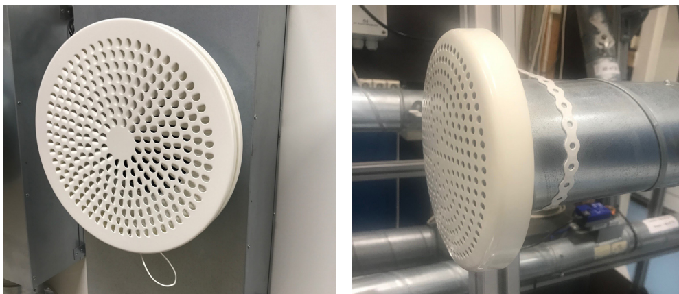
Examples of air terminal devices. Photo: SINTEF Community
