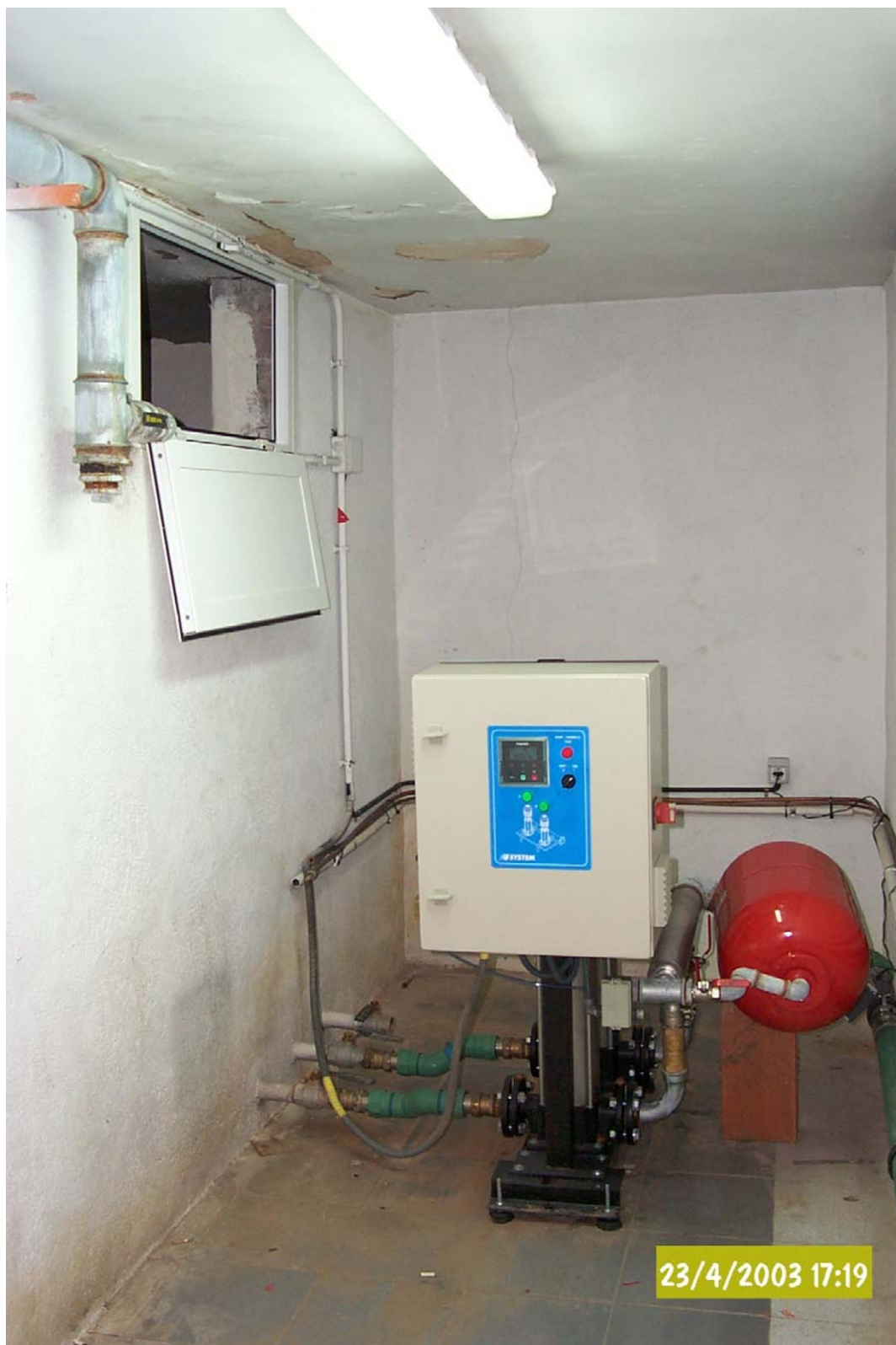
Figure 5 View towards water tank B and water pump for this tank (see Figure 1, floor plan). The photo was taken after the water tanks were completely separated.
