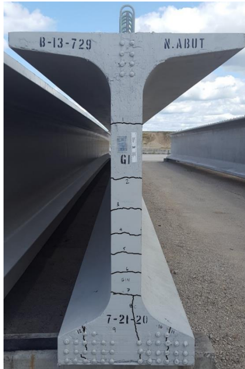
Figure 36. End region cracks in one of the girders from the field study. Lines are marked adjacent to each crack in the photo for emphasis.
