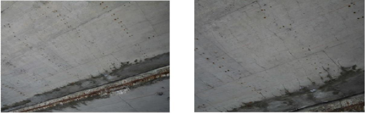
Figure 2. Photo of cracking in bridge under the deck (Figures from [7])
