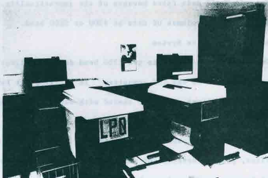
Fig. 4.3. Picture showing the 300 line per minute and 600 line per minute printers on the ATMOS PDP 11/34.
