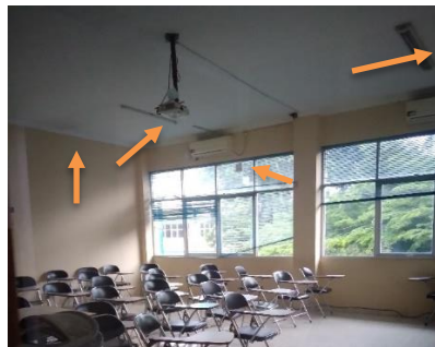
Figure 5. Structural and Falling Hazard Elements
