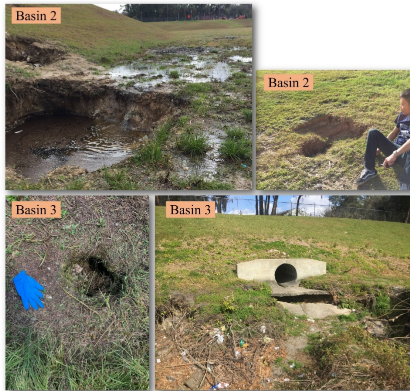
Figure 16. Open and collapsed sinkholes in Basins 2 and 3, observed during field surveys. Runoff was observed directly discharging into the local surficial aquifer through the open sinkhole in Basin 2. Photos were taken in Feb 2019 by Mohammad Shokri.
