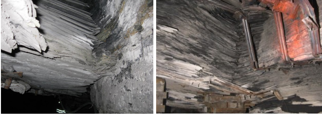
Fig. 1- 4 Cutter roof failure of shale roof (Molinda and Mark, 2010; Murphy, 2016)
