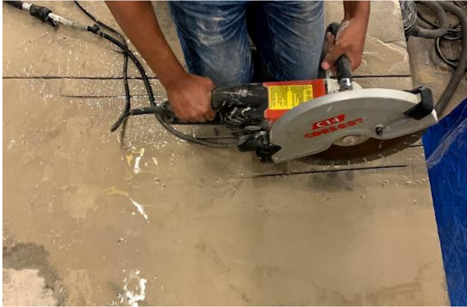
Figure 10.28: Concrete Deck Scoring
