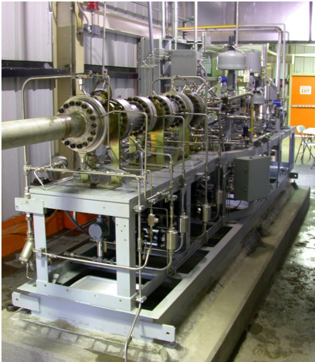
Clean Energy Systems' Oxy-Combustion 5MWe Gas Generator
