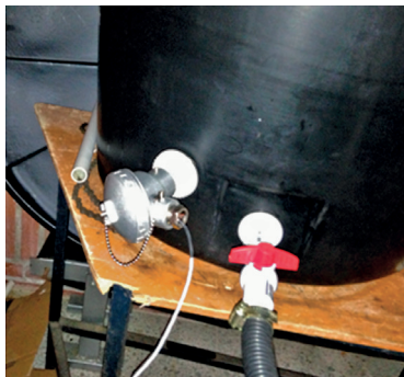
Fig. 2. Installed temperature sensor. Source: Authors
