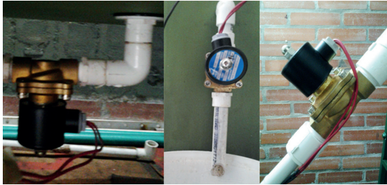
Fig. 11. Solenoid valves installed in the process. Source: Authors
