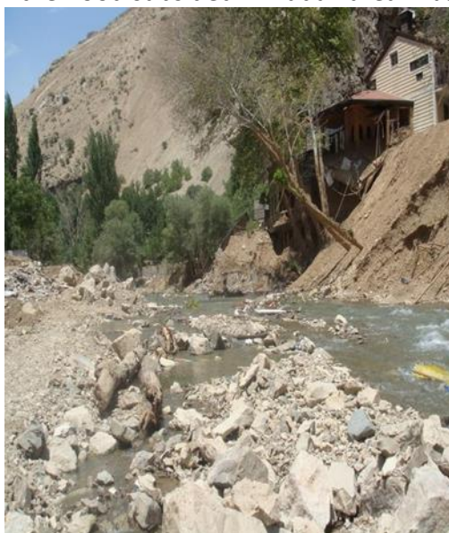
Figure 11 - Effects of river bank and villa demolition and accumulation of a large volume of bed load after the flood subsided in Rudak area in June 2018.
