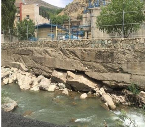
Figure 8. Erosion along the river at the site of Fasham refinery.
