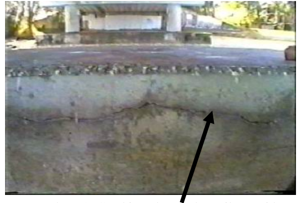
Photo 2. Cracking observed on pilecap sides
