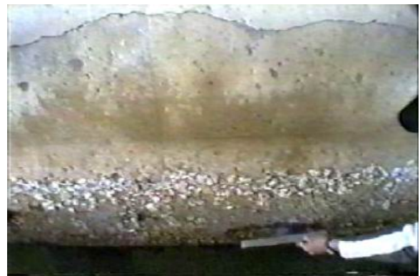
Photograph 4. Cracking and Spalling of concrete cover on sides of pilecap
