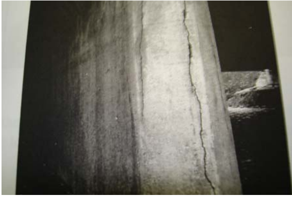
Photograph 5. Cracking observed on the chamfered edges of the pier.
