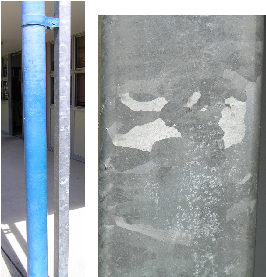
Figure 3.18. Galvanised post (right) and close up (left) showing signs of white corrosion product.
