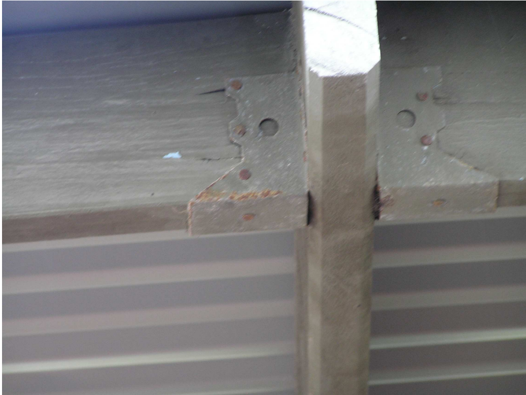
Figure 3.21. Gang nail plates showing some red rust and white corrosion product
