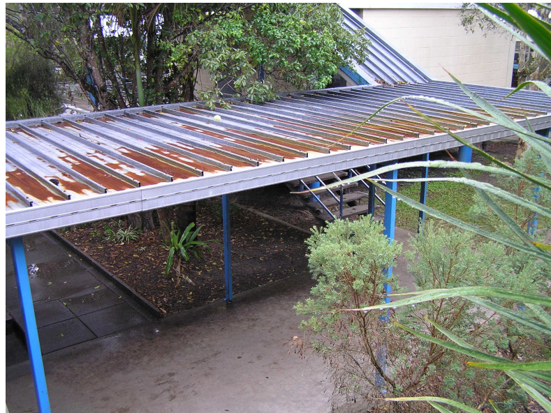
Figure 3.9. Galvanised Kliplok roof sheeting showing extensive red rust.
