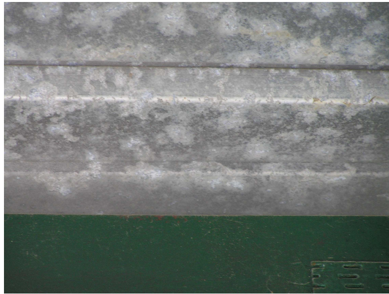
Figure 3.10 Underside of roof sheeting showing significant white corrosion product and some red rust.
