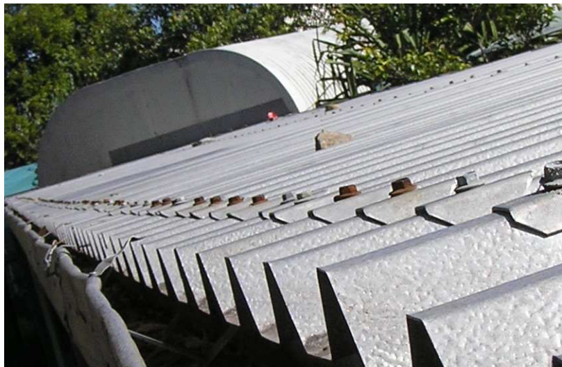
Figure 3.11 Heads of roof fasteners showing red rust and white corrosion product.
