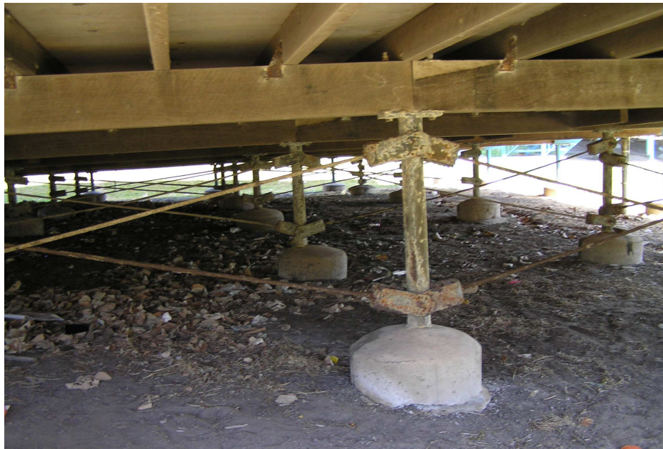
Figure 3.20. Significant deterioration of sub-floor metallic components on modular classroom.
