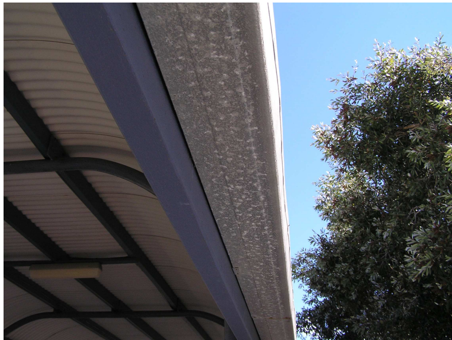
Figure 3.4 Underside of gutter showing significant corrosion.
