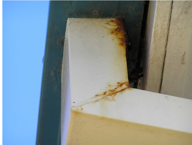
Figure 3.5 Rusting and deterioration on downpipe showing that problems are commonly associated with the joints.
