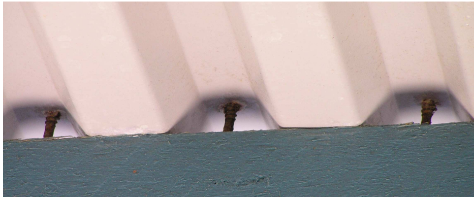
Figure 3.12 Fastener shanks showing red rust.
