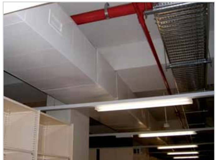
Services resolved: as built piping and ducting which were coordinated through the 4D model
