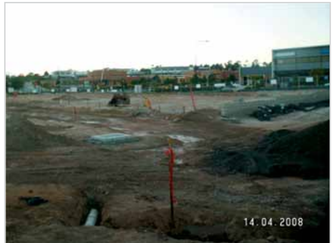
North Lakes Police Station site – before and at the start of construction
