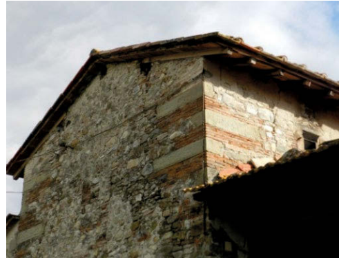
Fig. 5. Detail of the masonry at the corner of a drying room (Source: Mattone).
