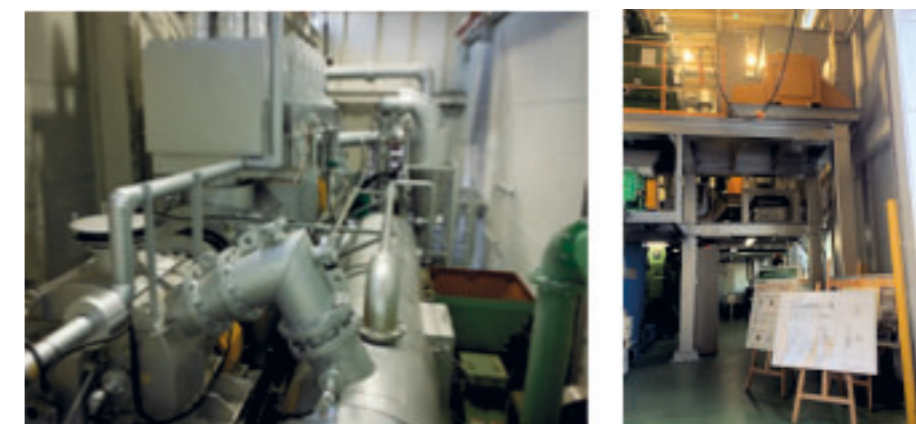
Demonstration plant for torrefied wood fuel, Isehara, Japan
