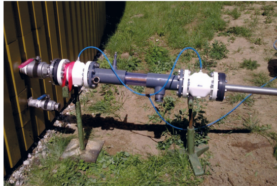
Figure 6.6-2: Example of a lock chamber for rinsing and sealing of the sensor (Source: TU Berlin)
