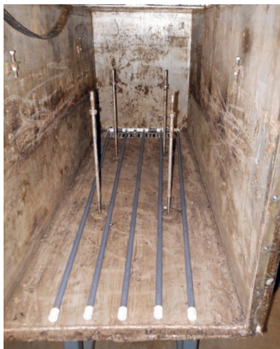
Figure 8.7-4: Aeration header in the base of the dry digester converted for use as an aeration bunker, the vertical rods for the substrate compression system are also visible (Source: InnoTech)
