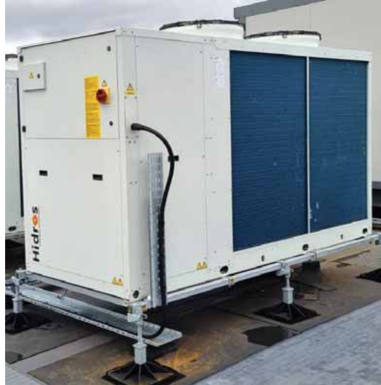
Hidros air to water heat pump installed at Sweeney's Corner student accommodation development.
