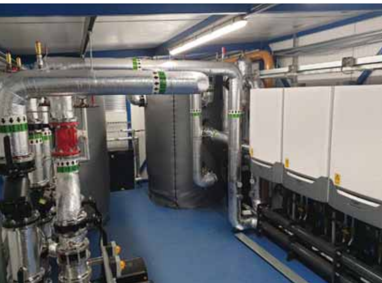
The Pak Plant packaged plantroom at Sweeney's Corner. Published by ARROW@TU Dublin, 2022
