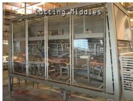
Figure 17. Middle cutting machine. The machine cuts off rib tops and separates the loin and belly automatically
