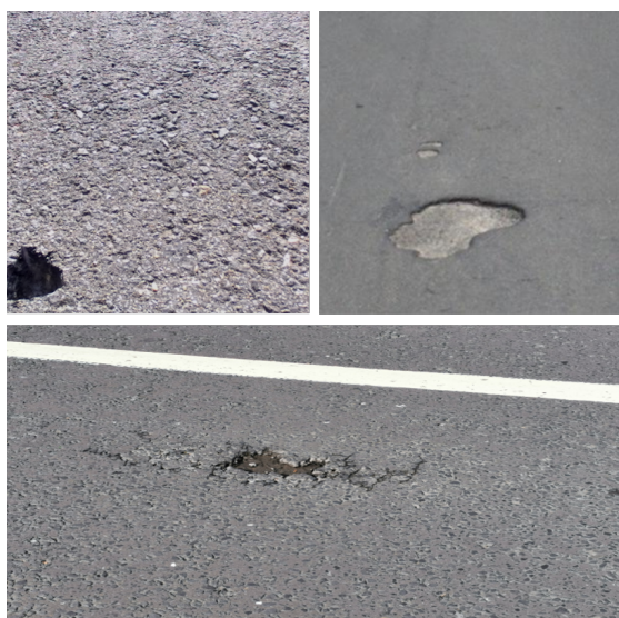
Figure 3: Example images of each testing dataset: Top left: Pothole-600, Top right: Cranfield Pothole Dataset, Bottom: Dublin Road Dataset.
