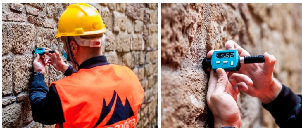
Figure 3. Non-destructive in situ survey with Equotip hardness tester on a masonry face of a building.
