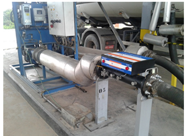
Fig. 10. Complete installation of the prototype in one of the HFO unloading terminals.
