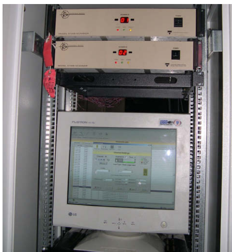
Fig. 10. Data acquisition system.
