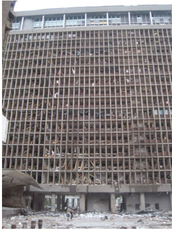
FIGURE 1: Terrorist attack in Oslo in 2011, failure of windows (from [5]).
