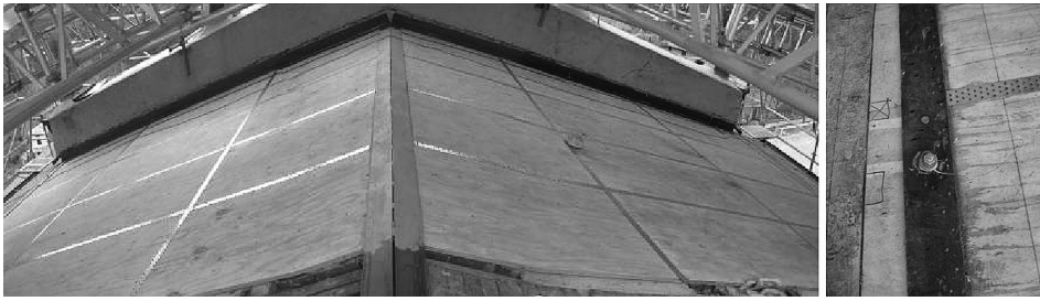
Figure 13. Photographs of the San Pietro Church in Roè Vociano: general view and of the plywood roof box structure and detail of the eaves chord connected to the underlying masonry by means of steel studs and deep anchorages.
