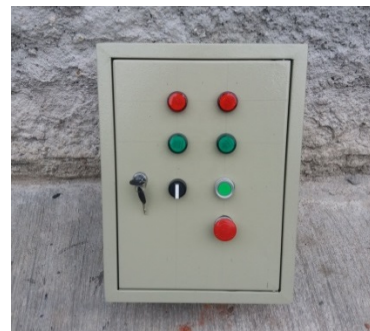
Gambar 14. Panel Control Cooling Tower
