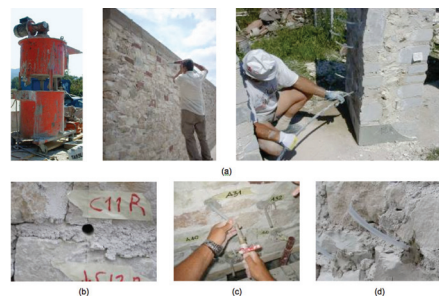
Figure 1. Grout injection procedure. (a) General overview of the process. (b) Drilling holes in mortar joints. (c) Fixing plastic pipes. (d) Injecting grout. (NIKER, WP3, Deliverable 3.2).
