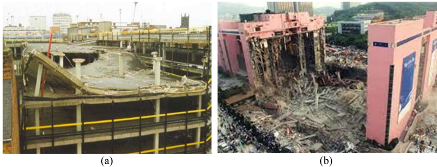
Figure 1 Flat slab failure worldwide: (a) Piper's Row Car Park, United Kingdom [7], (b) Sampoong Department Store, Seoul, Korea [8].
